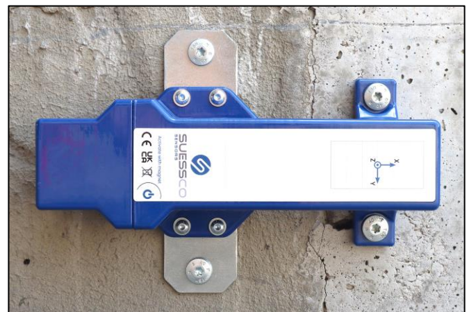
Reference crack application
