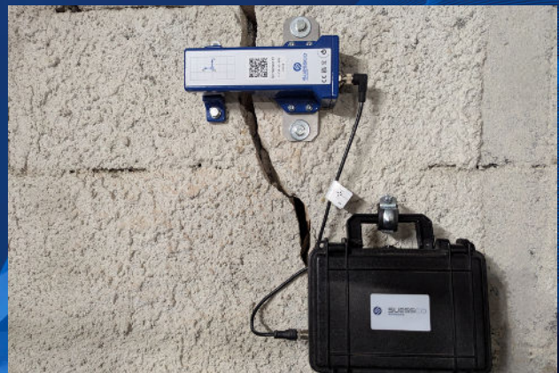
Reference Crack Application
