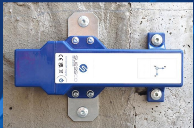
Reference Crack Application
