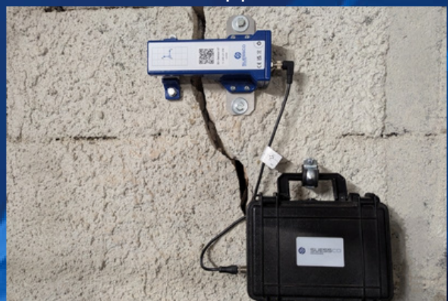
Reference Crack Application
